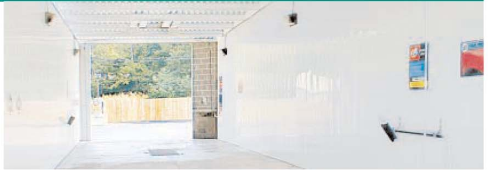
The brilliant white wall rehab using Extrutech PVC panels at the All Star Carwash has gotten rave reviews from Jimmy Allen's customers in Radcliff, Kentucky — "the bays now look like operating rooms!"
