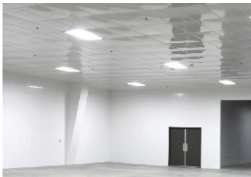
Drop Ceiling With Lighting
