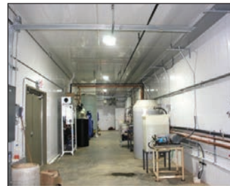
Car Wash Equipment Room
