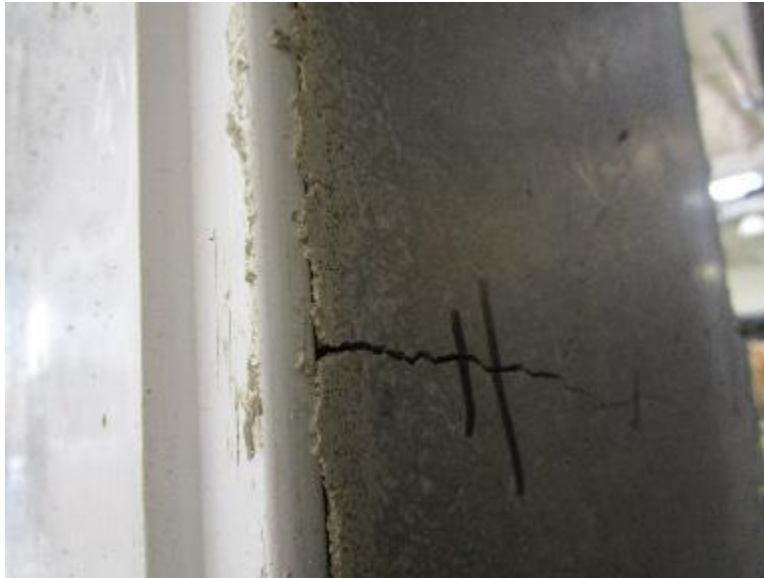
Photo No. 5 Transverse Load Test Panel Cracking
