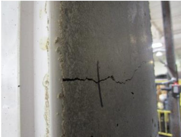
Photo No. 6 Transverse Load Test Panel Cracking
